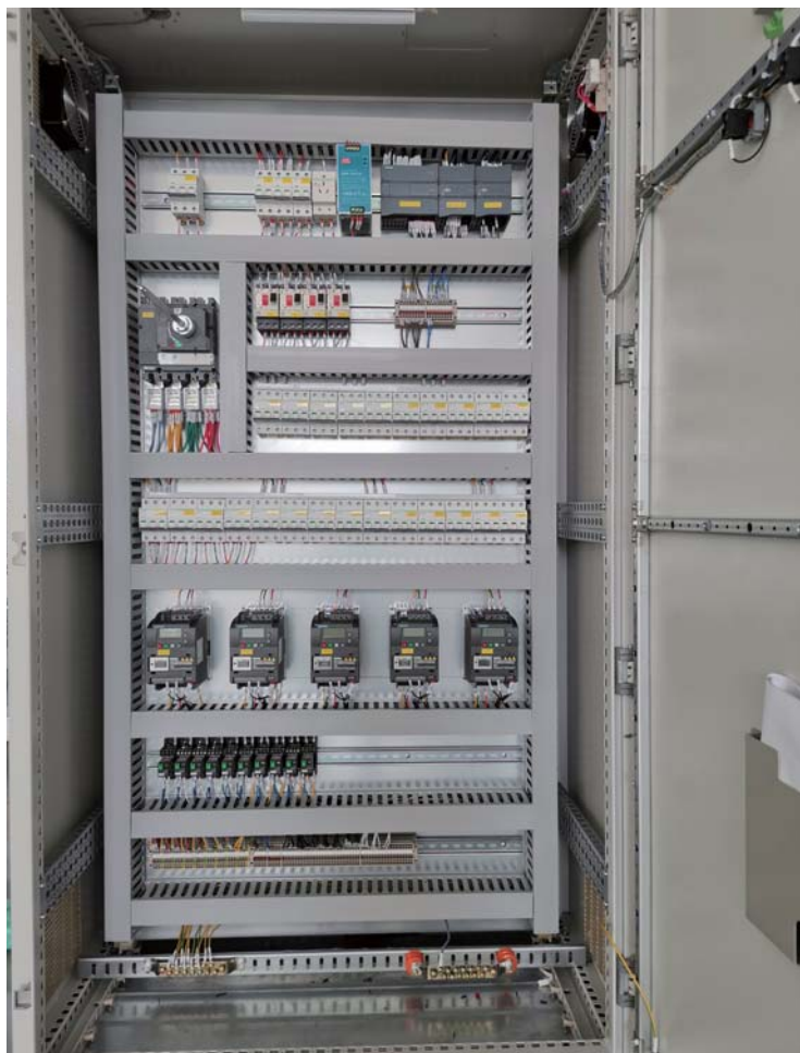
Electrical Control Cabinet 电控柜
